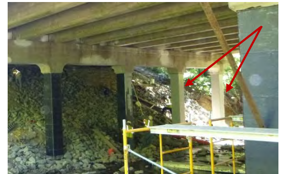
Figure 5: Sample Project with carbon fiber wrap designed by WRA. Notice the color coating on the two far right columns.
