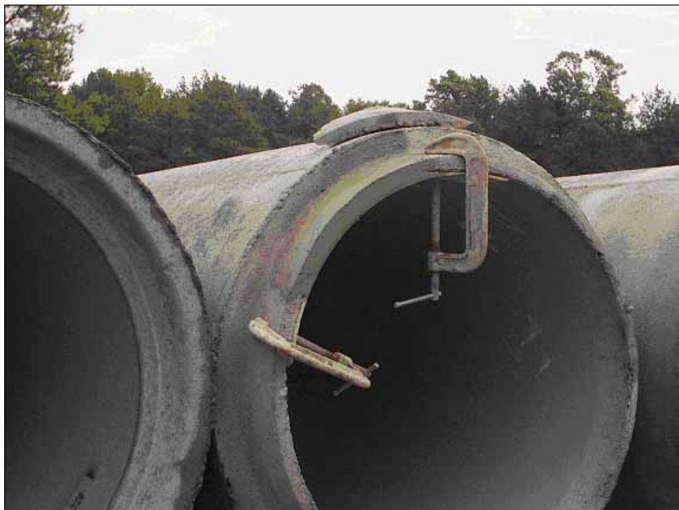
Photo 27 - Pipe with Patch
