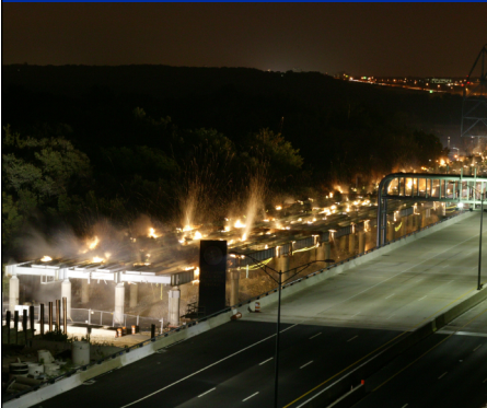
A nearly half-mile stretch of steel beams supporting the old Woodrow Wilson Bridge were detonated in the early hours of Aug. 29. "The Toughest Bridge Commute Contest" winner pulled the switch.
