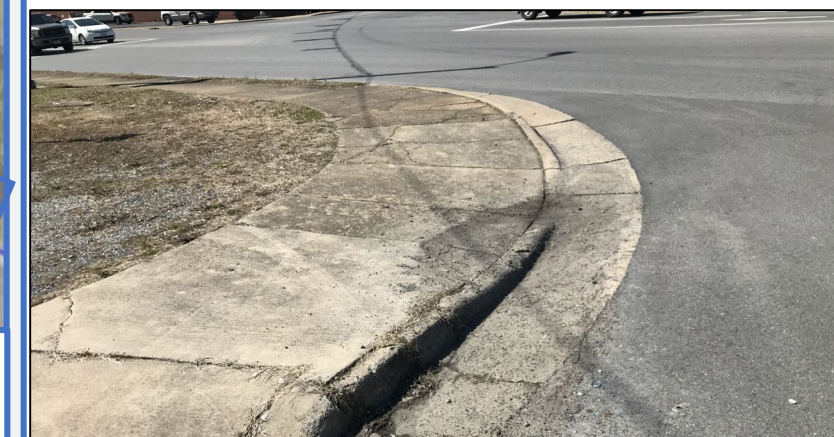
Non-ADA Compliant Curb Ramp
