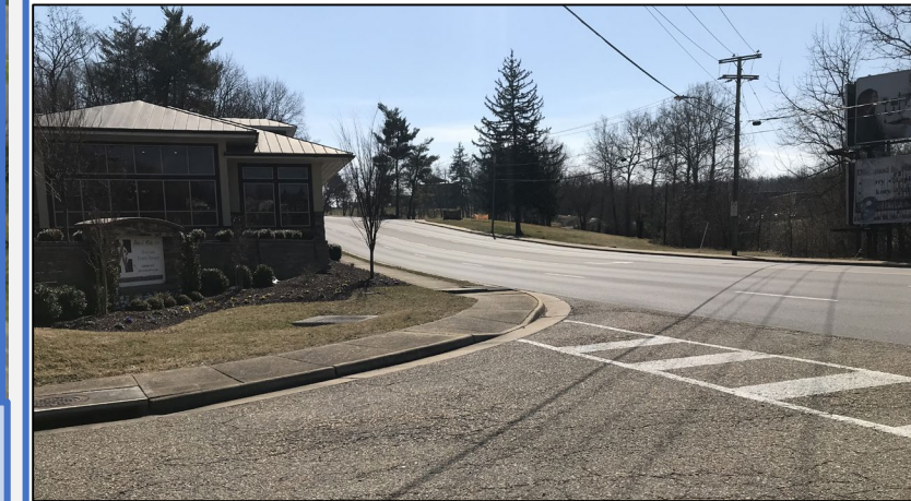
Non-ADA Compliant Curb Ramp
